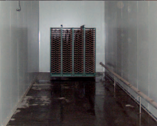
The drying chamber at Mediterran Kft. before (Fig. 1a), and after the upgrade by Kraft Energy (Fig. 1b)
