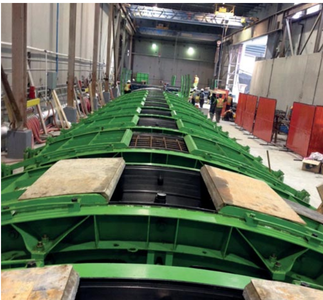
Evergreen Mold Segments cleaned and ready to pour concrete, molds are poured twice a day producing 48 segments a day which equals 6 tunnel rings.
