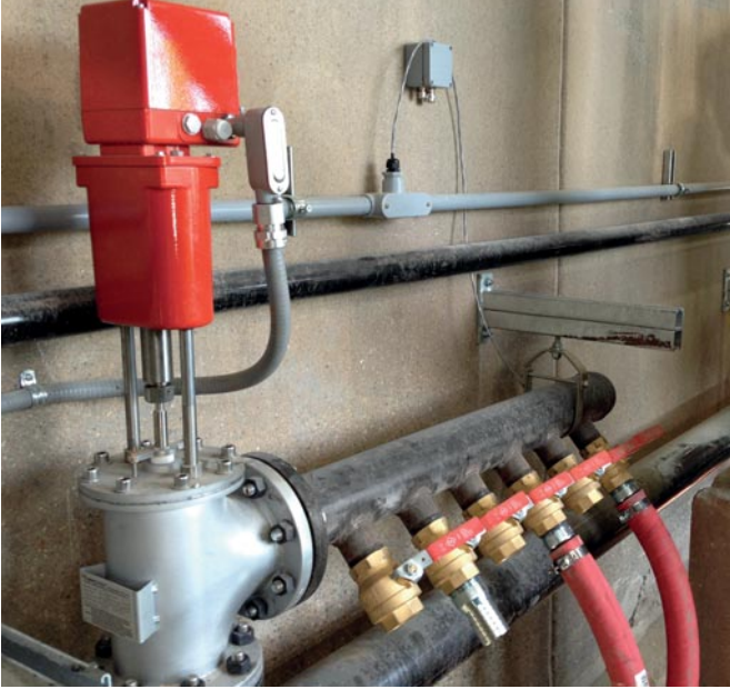
Vapor control valve with hose connections to inject vapor underneath the molds.
