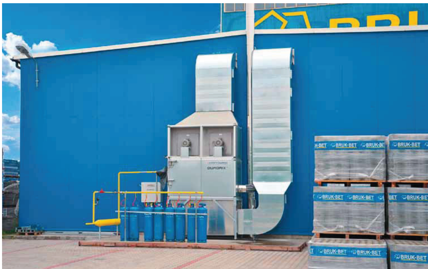
Figure: Kraft Curing Systems
