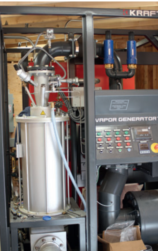
A single Kraft Vapor Generator (pictured during installation) supplies all curing enclosures of the Unistress production site with the optimal curing climate.
