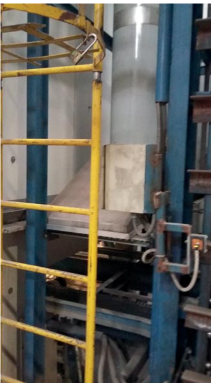
One of two heated hoods, installed between the lowerator and the exterior wall of the chamber, which prevents the escape of warm, moist air from the curing chamber and thereby prevents condensation dripping onto the fresh stones.
