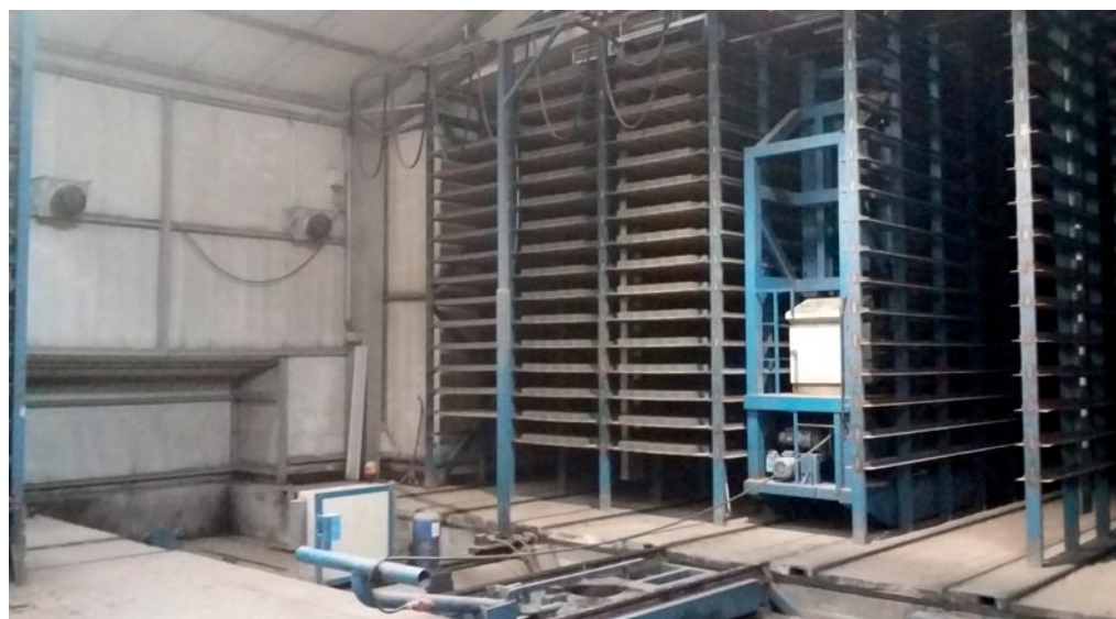
Thanks to the circulation of air in the transfer car area, both this area and the transfer car remain dry. No condensed water forms on the ceiling and there is no mist formation, which could lead to failure of the finger car's laser distance measuring system.
