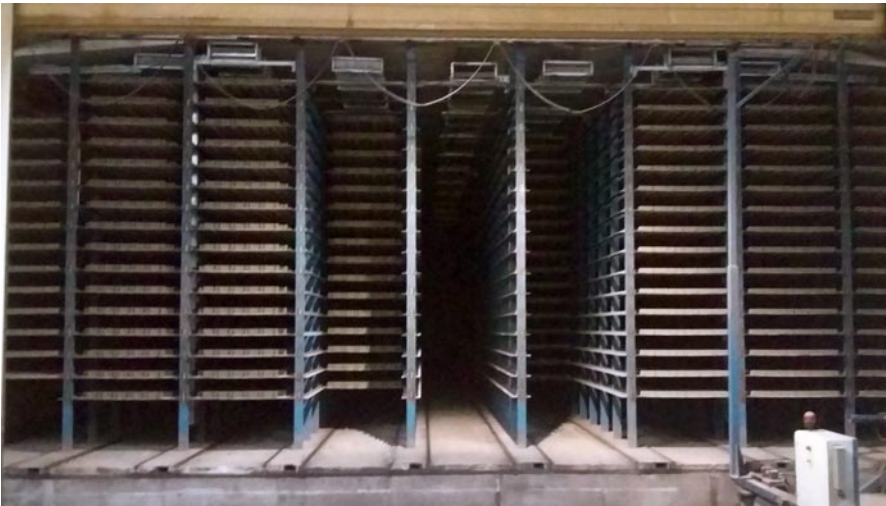
The galvanized supply and return ducts are mounted above the rack system. They don't take up necessary space. The floor is dry from front to rear in every corridor despite a humidity of 95 %.
