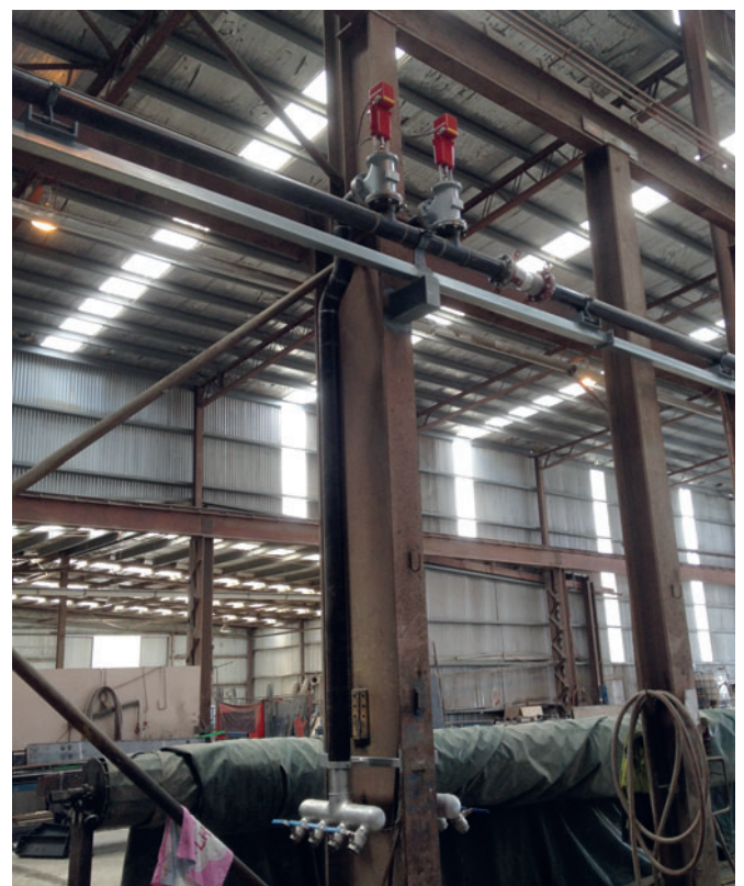
Fig. 4: Control Valves located throughout the production area control the flow of vapor automatically based on concrete temperature.
