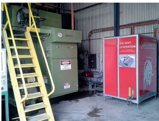
Fig. 3: The compact Kraft Curing KC 20-1S Vapor Generator (right) installed next to the boiler it replaced. Vapor Generators take up significantly less space than a conventional boiler of comparable output.
