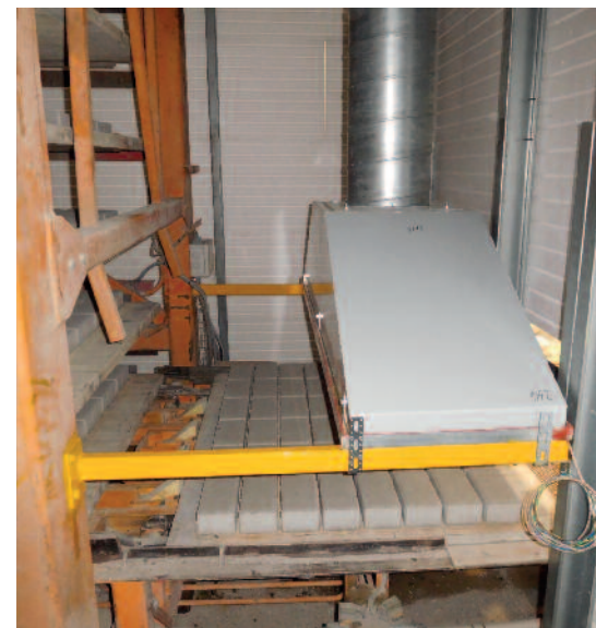
One of two heated hoods installed between the lowerator and chamber wall prevent the escape of warm and moist air, preventing any condensed drops of water reaching the fresh blocks.
