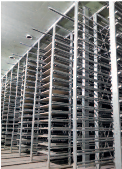
Air distribution lines inside the chamber to regulate air distribution and limit air velocity to less than 1.00 m/s.
