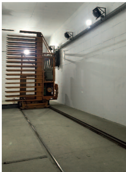
Due to the air distribution in the transfer table aisle, this area and the finger car remain dry. No condensate or mist forms that could result in a possible failure of the finger car distance measurement, which is carried out by lasers.
