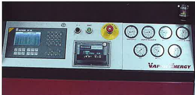
The control for the entire plant.
