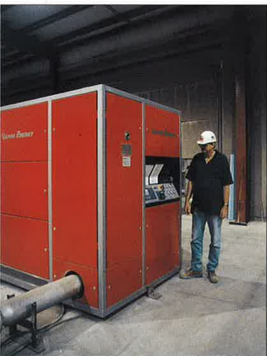
Small but wow! This small but almost inconspicuous unit supplies the whole Roaring Spring concrete works with energy for the after-treatment.
