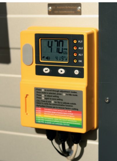
CO 2 sensors show CO 2 levels in the equipment room and concrete curing chamber
